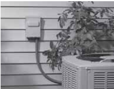
As an air conditioner disconnect
