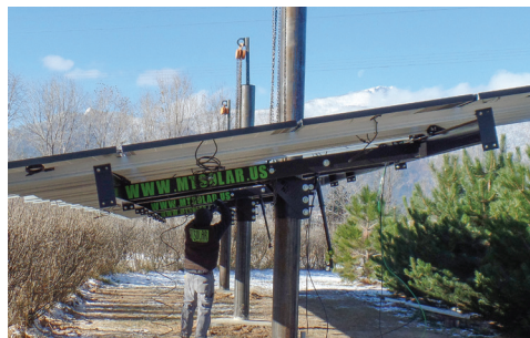
WIRE ON THE GROUND
