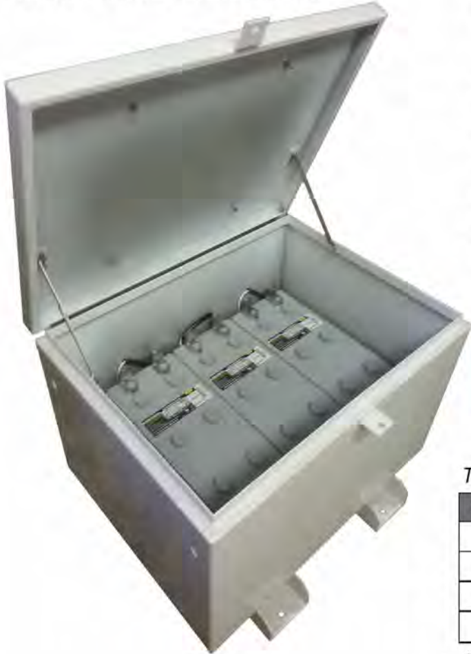
T-2X8D Enclosure with three 4D batteries
