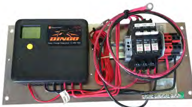
PRE Control Panel with a 20 amp DINGO
