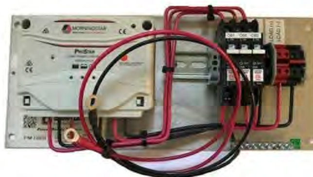
PRE Control Panel with a 30 amp ProStar
