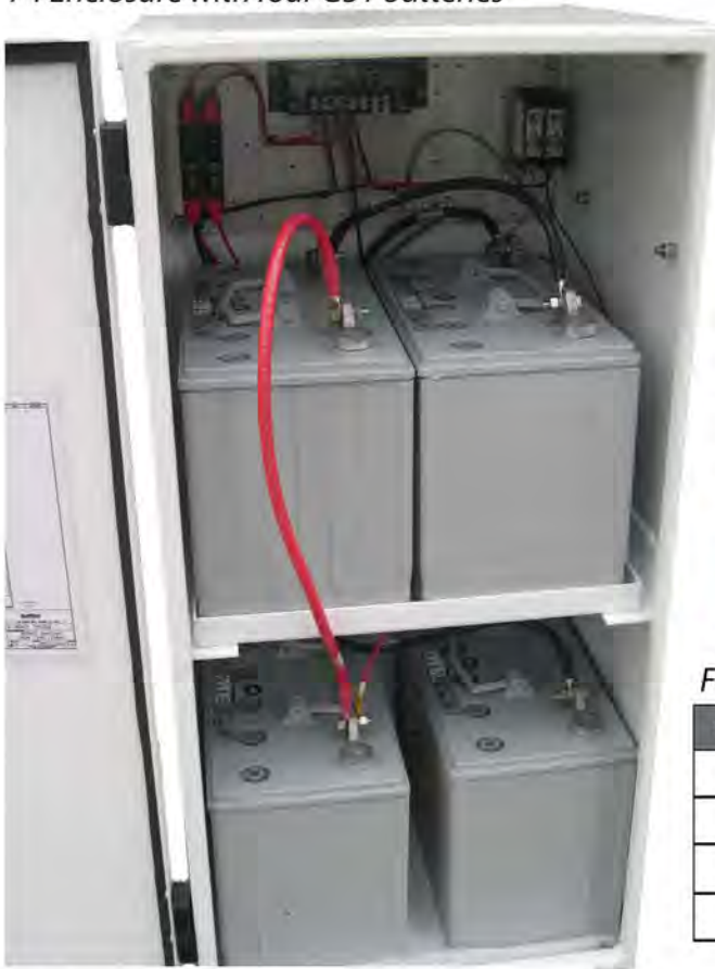
F4 Enclosure with four G31 batteries
